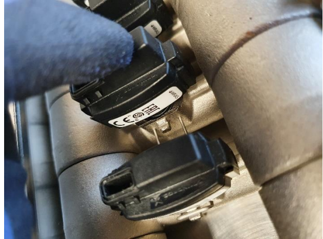
8. When the sensor is placed vertically, it can be pushed down into the piping
