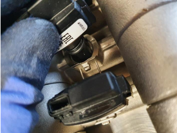
7. Insert the sensor gently in the piping.
